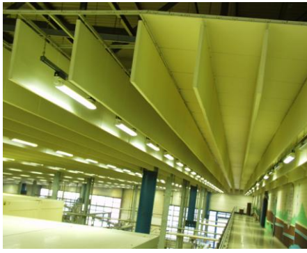
Figure 12: View to a baffle system above the plant
