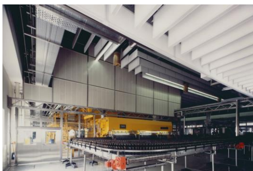
Figure 6a: Large washing machine in a bottling plant
